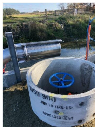
Bells Pond raw water intake screen
