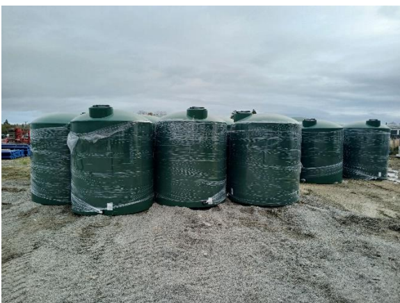
Mixed-Use Point of entry 5,000 litre tanks
